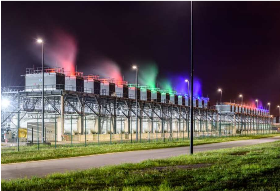
Google-colored lights illuminate steam rising from the cooling towers at our St. Ghislain, Belgium site.
